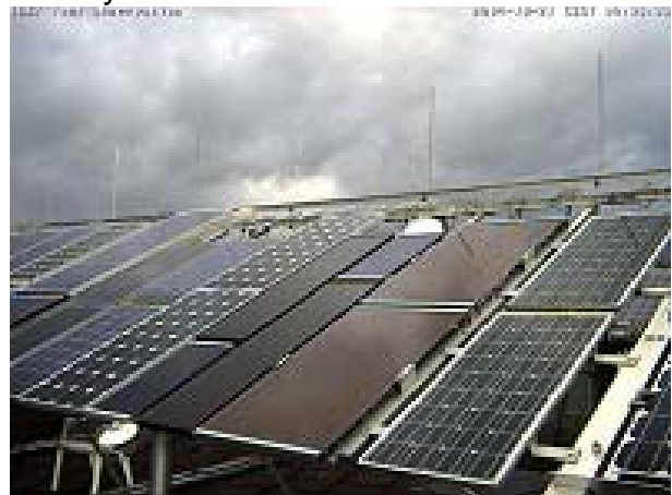
Fig 3 : Comparative module testing using MPP trackers at ISET in Germany
